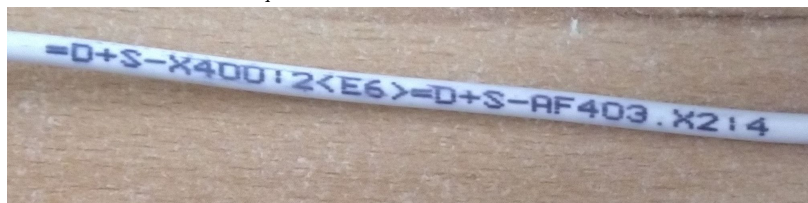
(c) Cable going from housing X400, slot 2 to housing row AF403, second housing, slot 4
